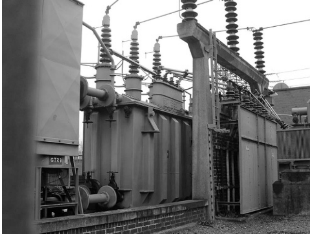
Figure 5.2 Transformer: 132 to 33 kV. (Courtesy of Murray Thomson)
