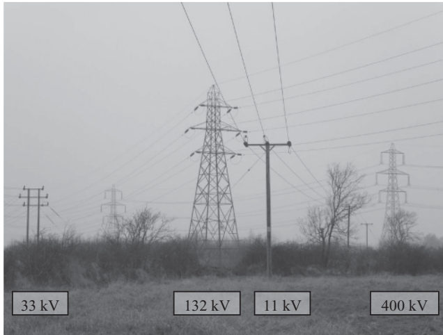
Figure 5.1 Overhead lines at four different voltage levels. (Courtesy of Murray Thomson)
