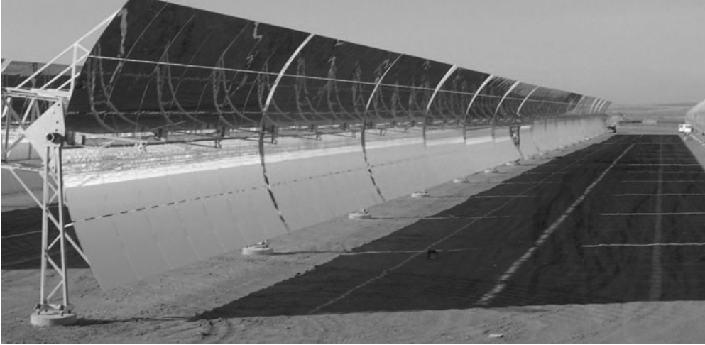
Figure 2.16 50MW parabolic trough plant with thermal storage at Andasol, Spain. (Reproduced from Concentrating Solar Power – from research to implementation. © European Communities, 2007)
